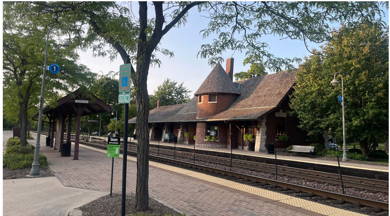
Photo of the Metra Station area shows unit pavers in need of replacement.
